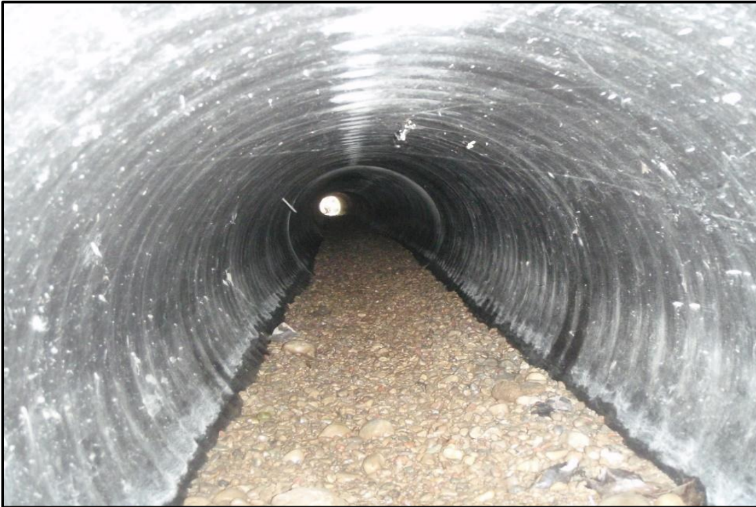
Photograph 8. Example of Substrate Placed on Culvert Bottom to Promote Wildlife Passage
