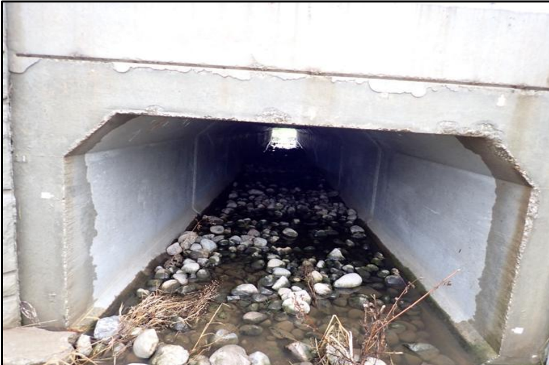
Photograph 5. Example of Substrate Placed on Culvert Bottom to Promote Wildlife Passage
