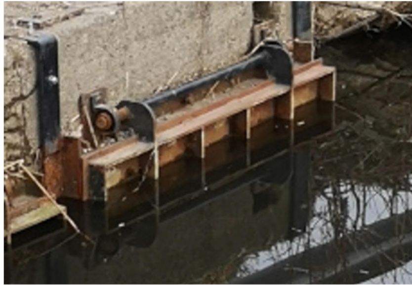
Figure 17 Point Abino Outlet Flap gate
