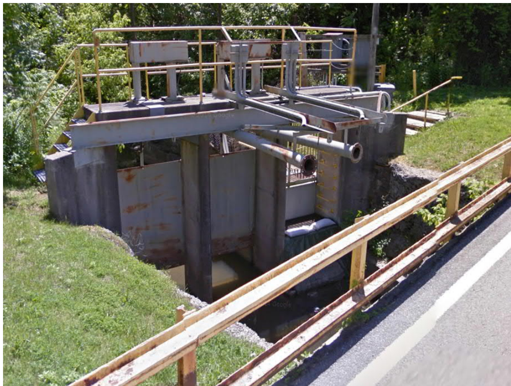
Figure 32 Wignell Control Structure - 01
